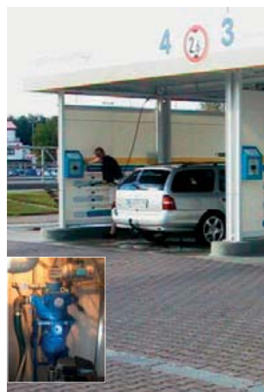
Car-wash water preparation with an automatic filter and bioreactor
